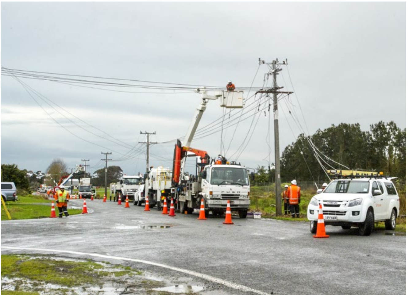
Reconductoring project to replace end of life assets in central Dargaville including undergrounding a portion of the 11kV line to improve reliability and resiliency.
